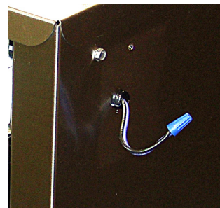
Figure 7: Control connection wires.
